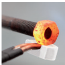
Releasing of rusted bolts
